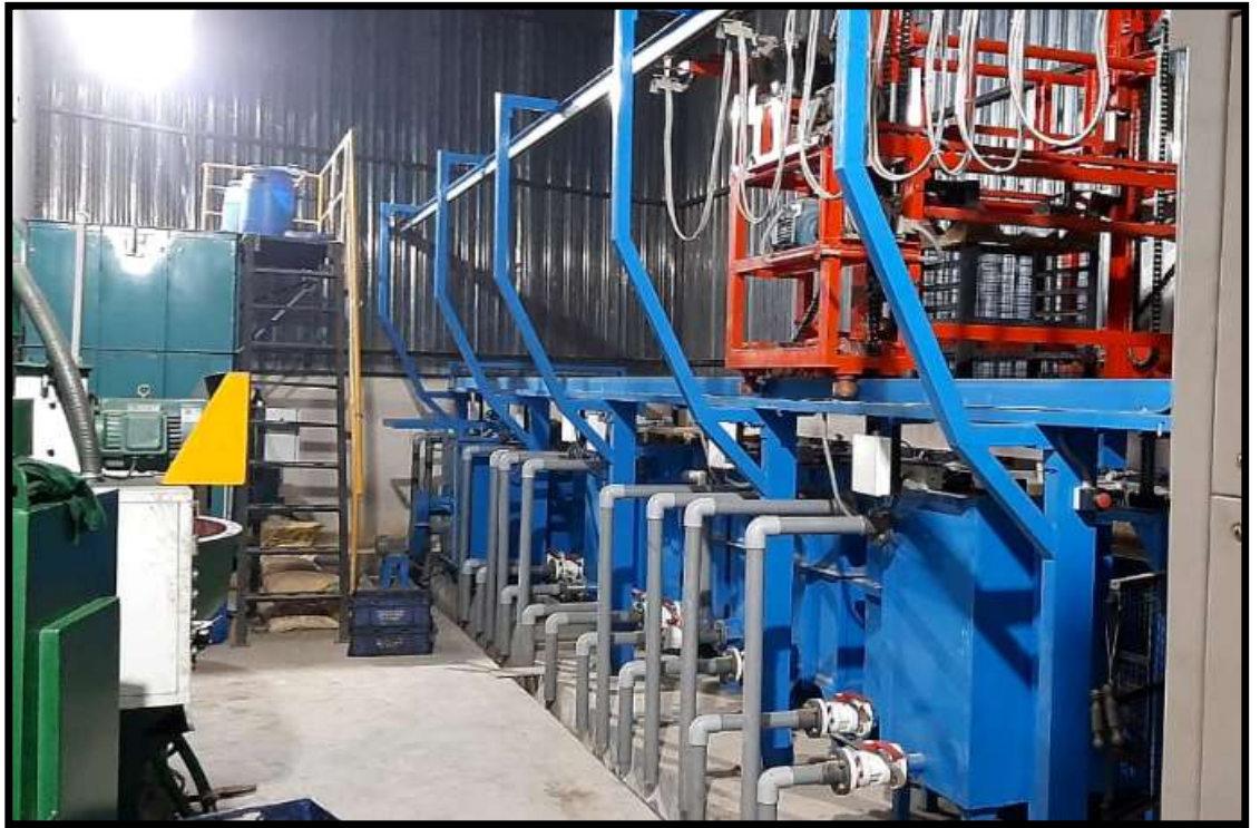
Conveyorized Manganese phosphating plant
